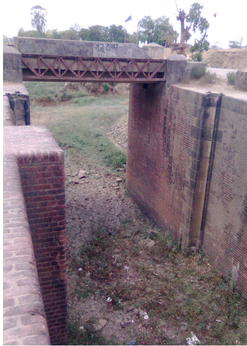
Lock of the canal as it enters Buxar town; like the rest of the canal, it's dilapidated
